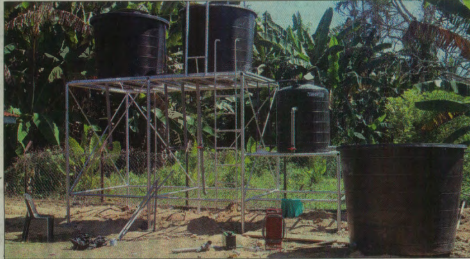
The micro water treatment system built by the academicians for villagers of Kg Merabau.
